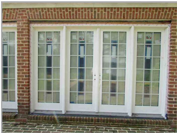
Exterior view of French doors in family room. Doors show missing hardware and trim work.
