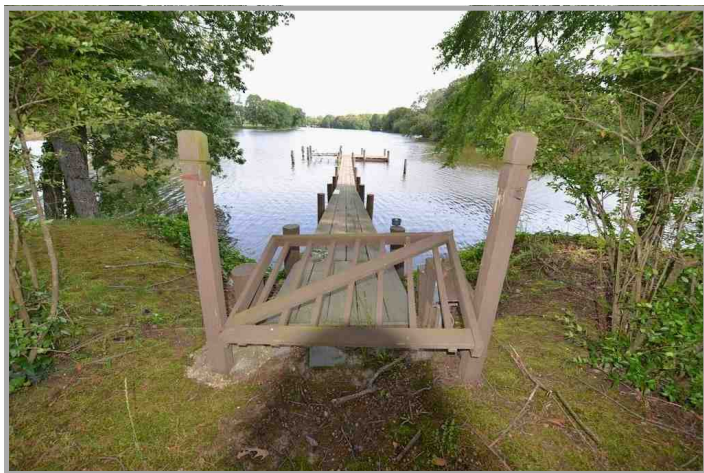
View of broken gate at Subject dock. Subject is located at the head of Pickering Creek.
