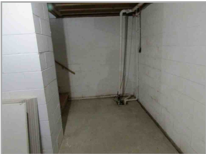
Sump pump in basement.
