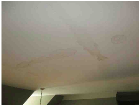
Possible Water Damage
