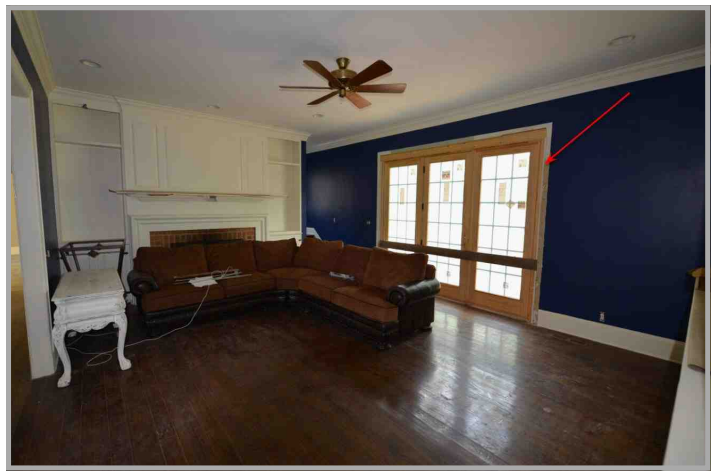
Family room showing custom built ins, fireplace, wide ceiling molding and ceiling fan. French doors show missing trim and hardware.
