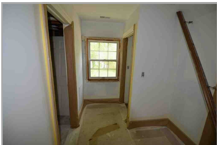
View of missing window jamb and light switch plates.
