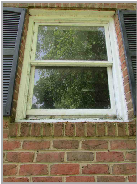
Exterior wood shows peeling paint.
