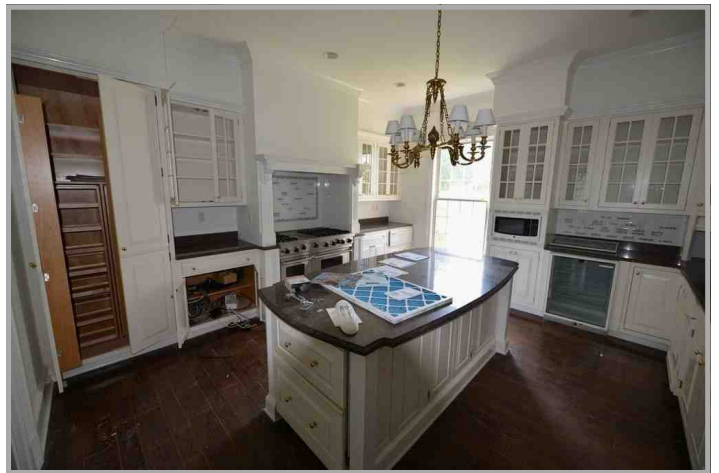
Kitchen showing quality moldings, cabinets and fixtures. High end stainless Viking gas stove. Kitchen appears functional.
