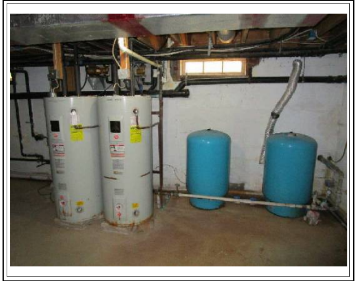
Basement - HWH/Pressure Tanks
