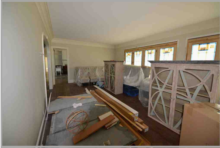
Living room shows French doors missing hardware, door jamb and trim work.
