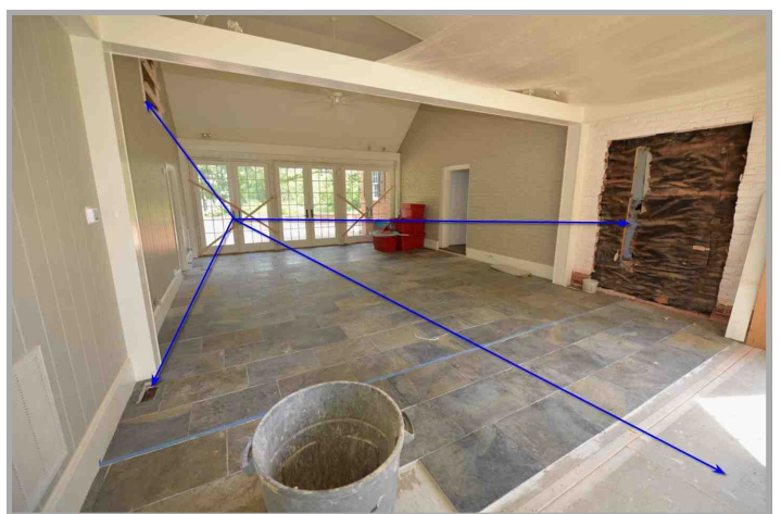
Breezeway is under construction showing exposed laundry room to the right, missing floor lower right, missing register lower left and open wall to living area over garage.
