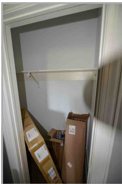
Closet in foyer shows missing door.
