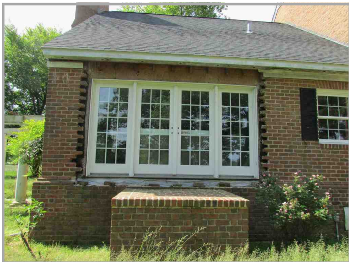
Exterior view of French doors to master bedroom. Doors show missing bricks along door jamb and header.
