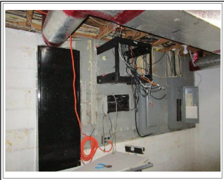
Basement - Electric Panels
