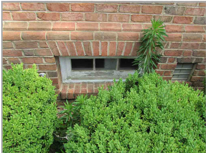
View of basement window. Exterior wood surfaces show peeling paint.
