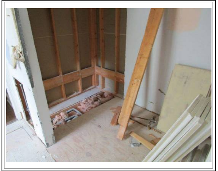
Full Bathroom #3 - Photo #2
