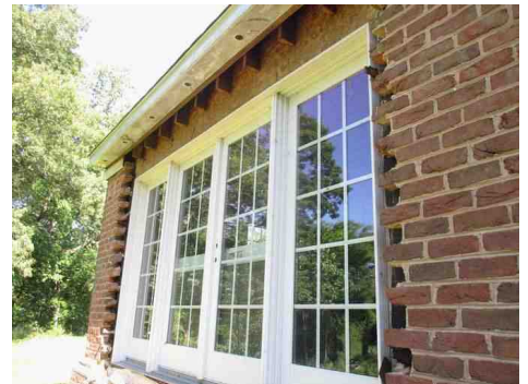
Unfinished Door Frame
