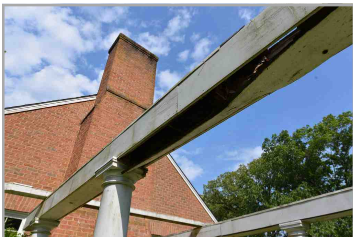
Pergola is weathered and shows rot.
