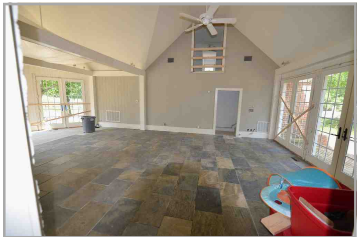
View of breezeway to garage. Breezeway is heated and cooled space, and included in estimating GLA.
