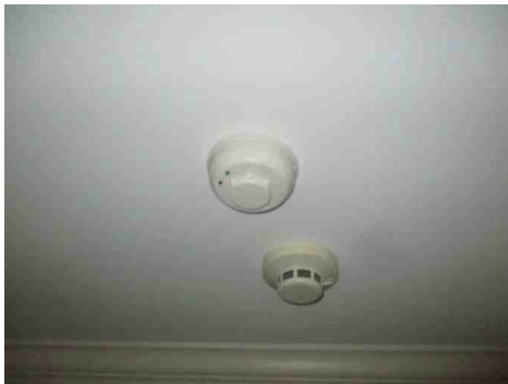
Smoke / CO Detector
